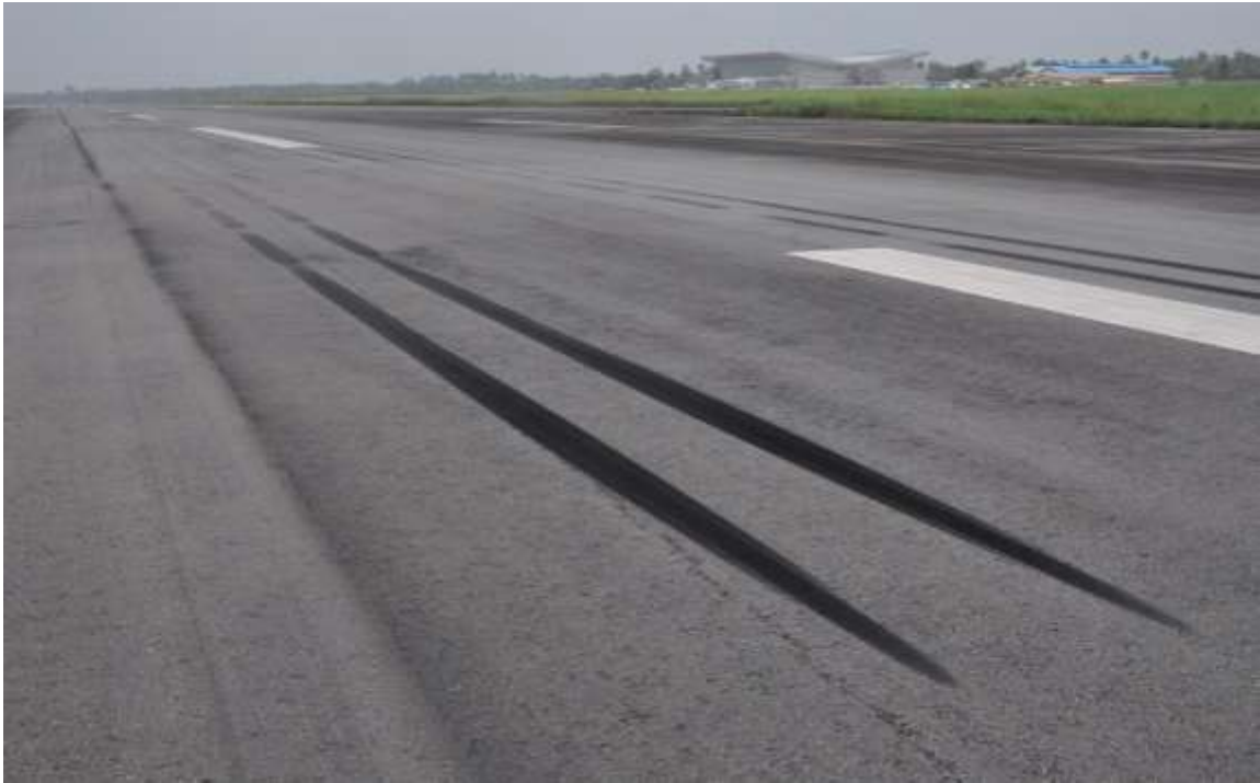
Figure 4: Picture showing skid marks on the runway
